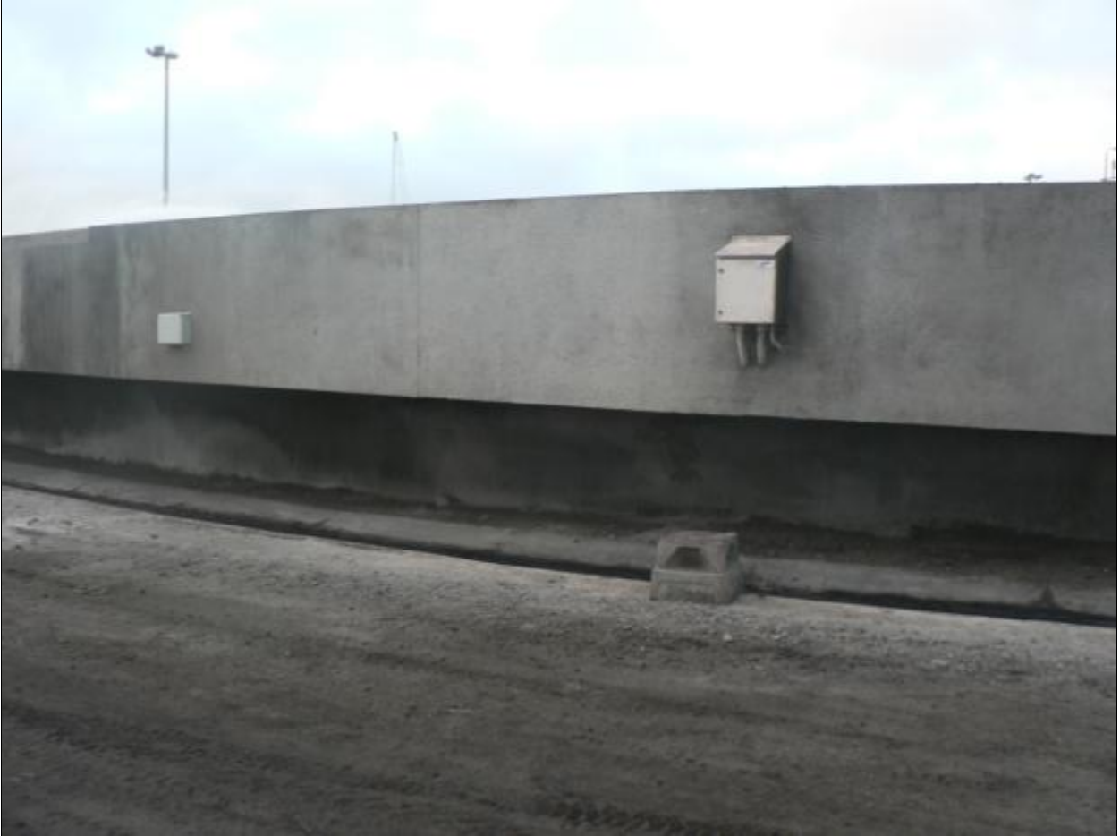
Completed Tank Concrete Surface showing monitoring and junctionboxe.
