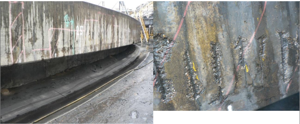
Corroded Reinforcement causing concrete spalling in the external launder wall of the tank
