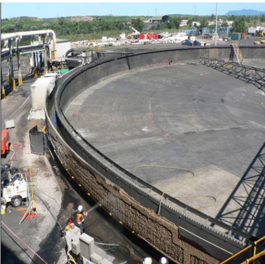
Coal Thickener Tank during 2 week shutdown. Hydro-demolition & dry process gunite progressing around the tank.
